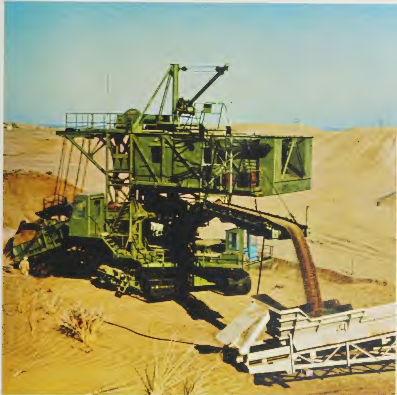
16 In the extensively mechanized production from marine deposits, the most modern machinery is employed to shift the huge quantities of sand.
