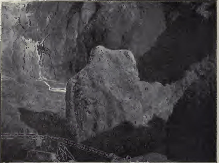
Mount Ararat before Blasting. (Removal of a piece of "Floating Reef," Bultfontein Mine, 1901. It was 150 feet long, 50 feet wide, and 120 feet high. 180 holes were drilled in it and charged with 1050 pounds of No. 1 dynamite.)
