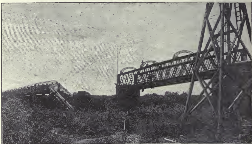
Railway Bridge over the Vaal River at Fourteen Streams, destroyed by the Boers.
