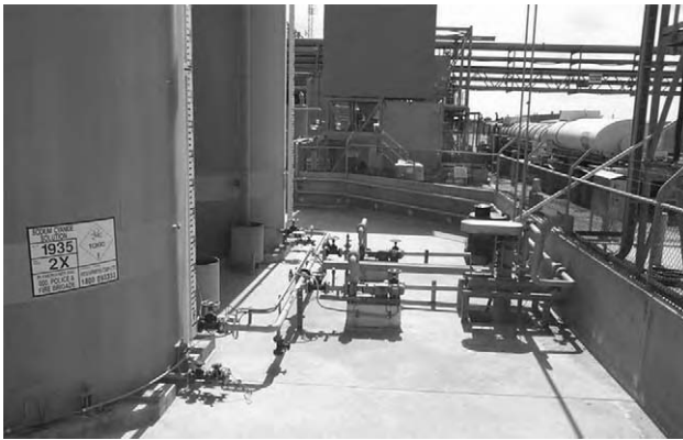
Fig. 7. Liquid cyanide storage tank and bund.
