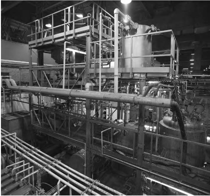
Fig. 3. The HSSE plant.
