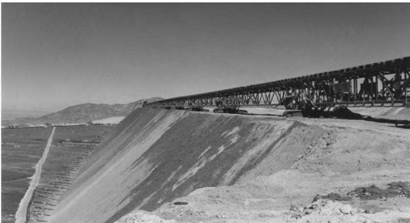
Fig. 4. Rahco stacker building a 12 m lift by tripping the ore over the advancing edge. The stacker can climb ramps and turn sharply to fit project requirements.
