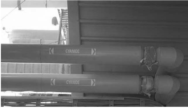
Fig. 6. Cyanide pipe colour coding and flange guards.
