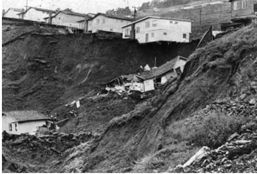
FIGURE 5 Houses in Oakland, California, destroyed or damaged by a deep-seated landslide in 1958 after an unusually rainy winter (Oakland Tribune photo).
