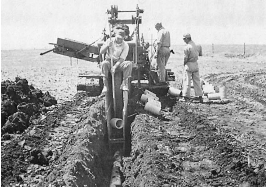
Figure 14–13 Concrete tile being placed with tiling hooks behind a trenching machine. (Courtesy W. H. Lathrop.)
