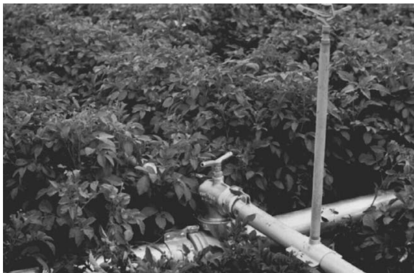
Figure 15-11 A sprinkler at the top of a riser on a portable line in a potato field. Water strikes the protruding arm and makes it work back and forth against a spring. This action rotates the sprinkler head and helps distribute the water. (Courtesy F. R. Troeh.)
