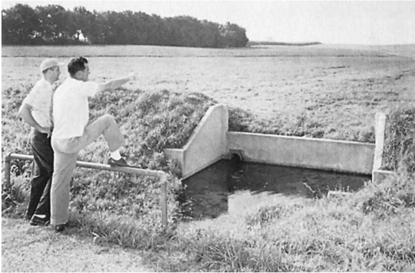
Figure 11–12 A concrete drop structure that serves as an outlet for a grassed waterway. The round hole visible in the lower left corner of the structure is the outlet for a tile drain that reduces the time the waterway stays wet. (Courtesy USDA Natural Resources Conservation Service.)
