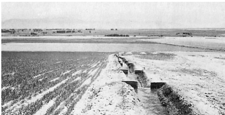
Figure 15-7 A series of drop structures protecting a ditch in Idaho. (Courtesy USDA Natural Resources Conservation Service.)
