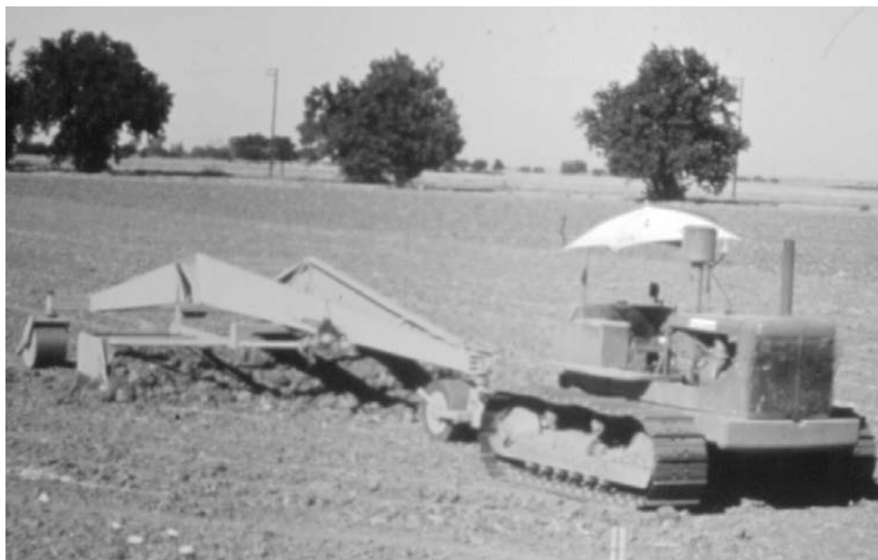
Figure 15-16 A land plane is used to smooth land surfaces for more uniform surface irrigation. (Courtesy F. R. Troeh.)
