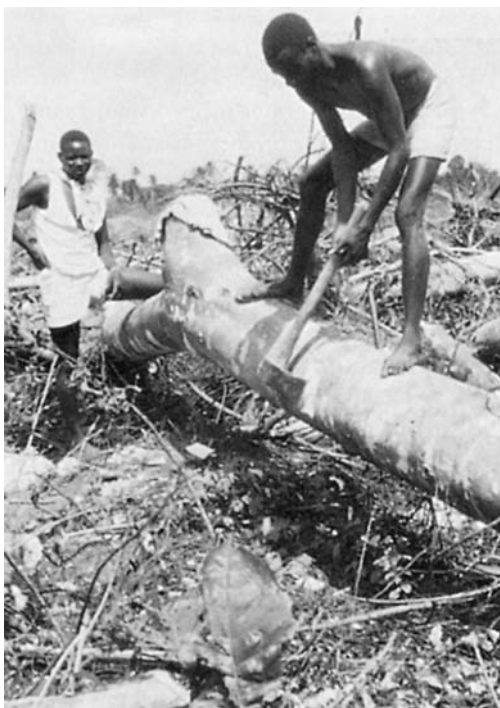
Figure 20-2 Shifting cultivation on forested soils requires that a dense stand of trees be cut down and burned. Bulldozers have been used experimentally, but they cause serious soil deterioration. Much of the work is done with an axe, as shown in this scene in the Ivory Coast. (Courtesy Roy L. Donahue.)
