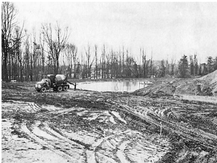
Figure 11-1 Sediment from this construction project in West Virginia would pollute the nearby stream if it were not caught in this debris basin. (Courtesy USDA Natural Resources Conservation Service.)
