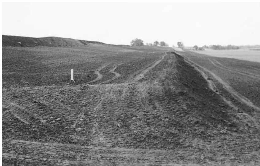
Figure 10-3 A newly constructed steep backslope terrace in Iowa. This terrace is straight and parallel to the fence line. The near end of the channel is blocked and the water drains through a white, vertical pipe at the bottom of the channel into an underground pipeline. (Courtesy F. R. Troeh.)
