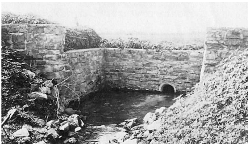
Figure 19–2 A masonry drop structure and tile outlet built by the Civilian Conservation Corps to prevent a gully from advancing up this Iowa waterway. (Courtesy USDA Natural Resources Conservation Service.)
