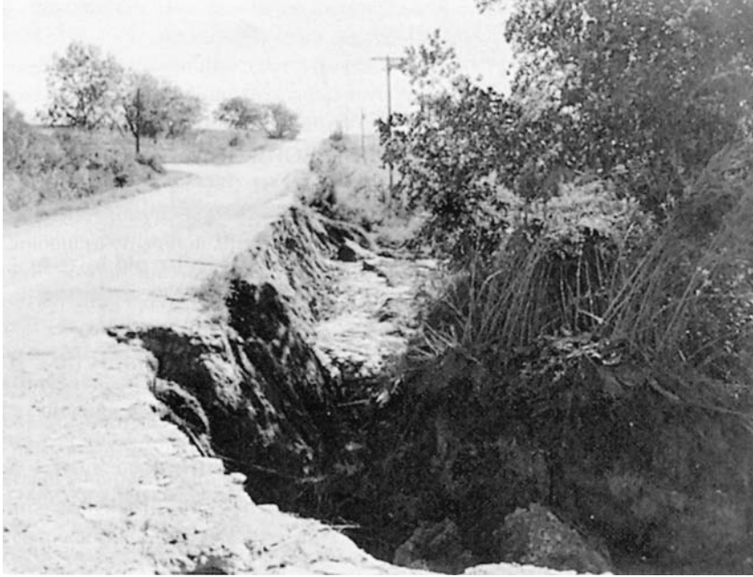
Figure 4-4 Erosion damage to the ditch along a roadway in Kansas. (Courtesy USDA Natural Resources Conservation Service.)
