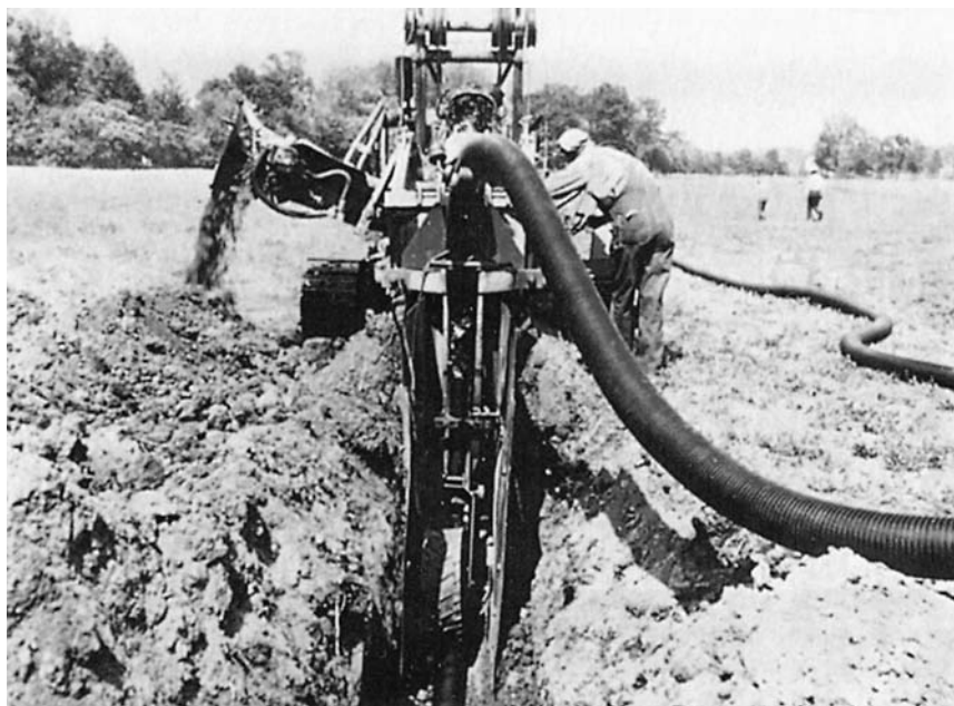
Figure 14-14 Flexible plastic tile being installed by a tiling machine. (Courtesy USDA Soil Conservation Service.)
