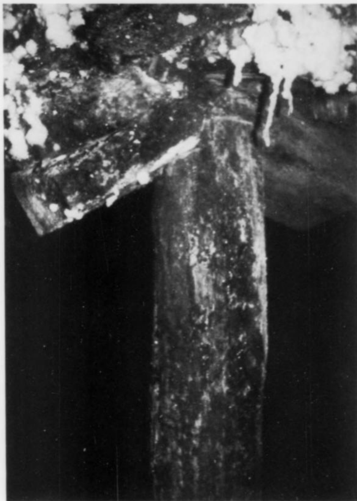
Figure 6. Decomposing underground timbers encrusted with halite and thenardite. Photo by Stan Celestian.
