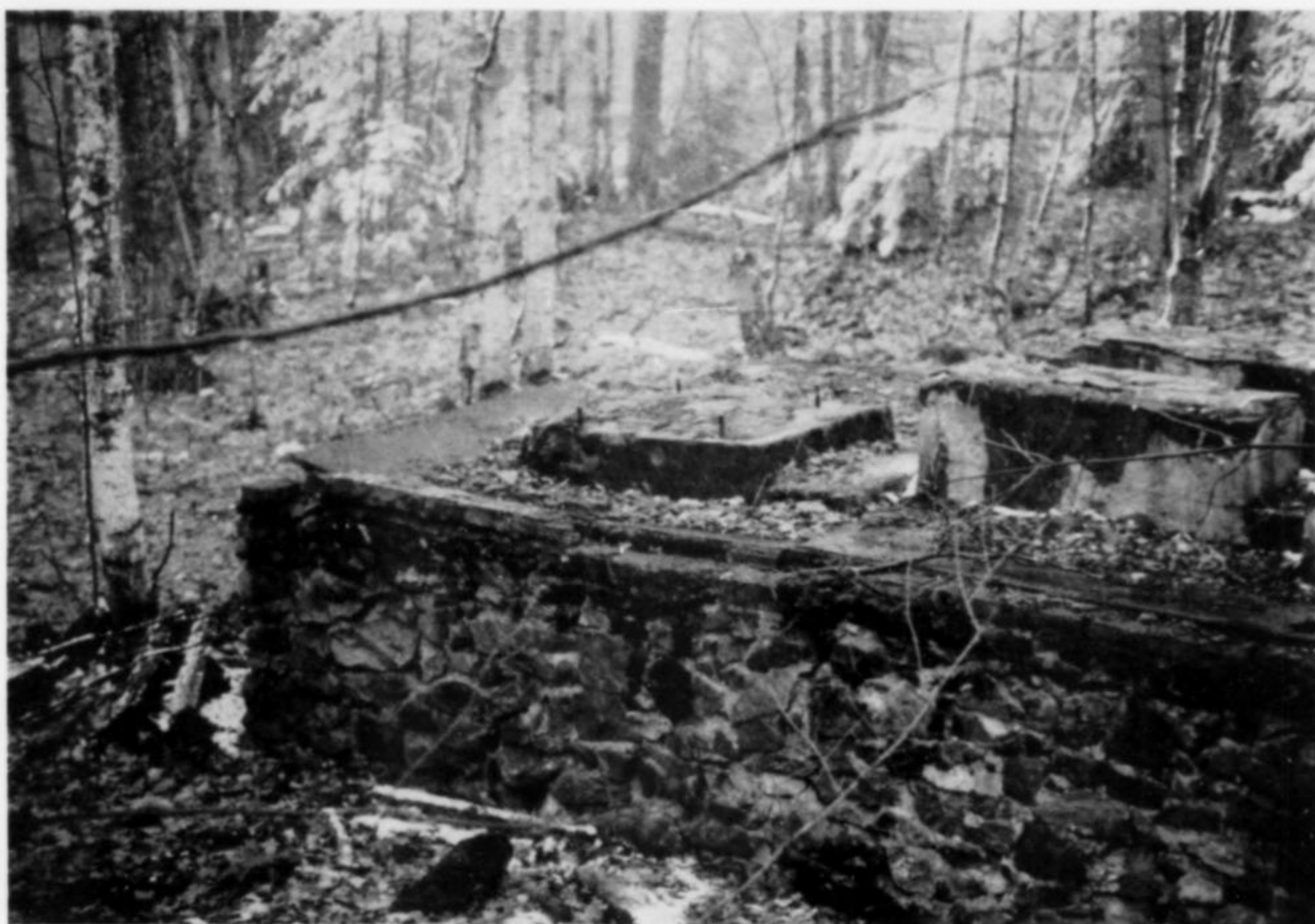
Figure 5. Decaying foundations near the Ropes mine today. Extensive dumps are located nearby.
