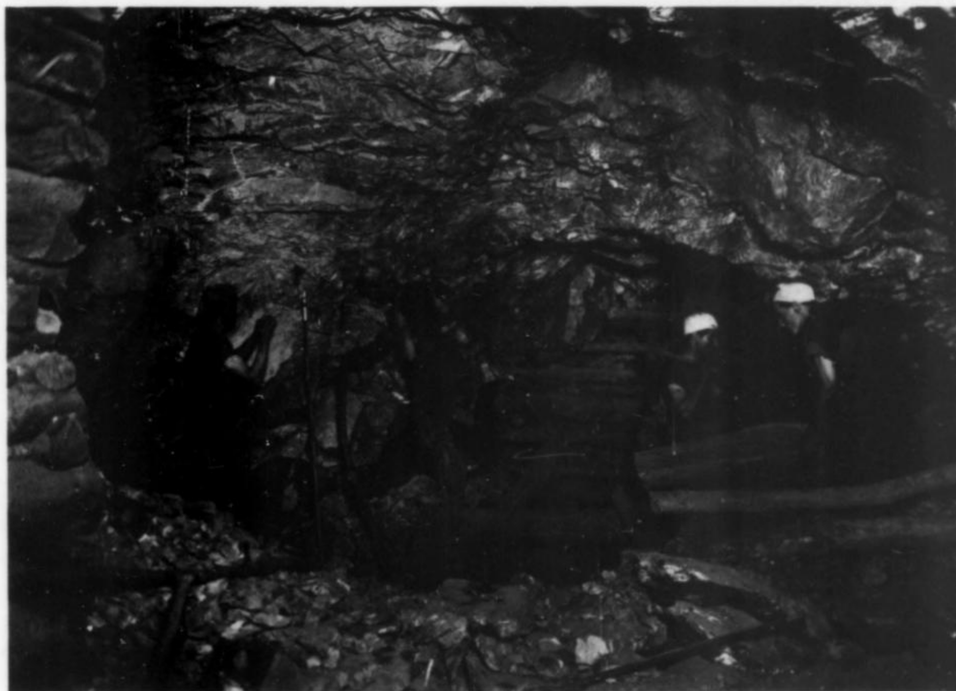
Figure 10. Working a wide stope at the Wallaroo mines during 1916–1918. The stope was worked by a tribute team of four with four laborers to assist with timbering. (SADME 7167)
