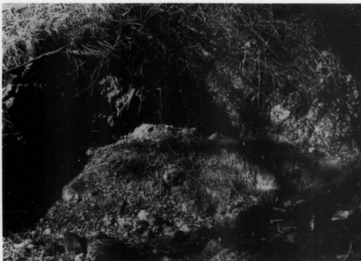
Figure 5. View of one portal of the Stayton mine which had not been closed; extensive caving was noted within 10 meters of the portal. G. Dunning photo, 1987.
