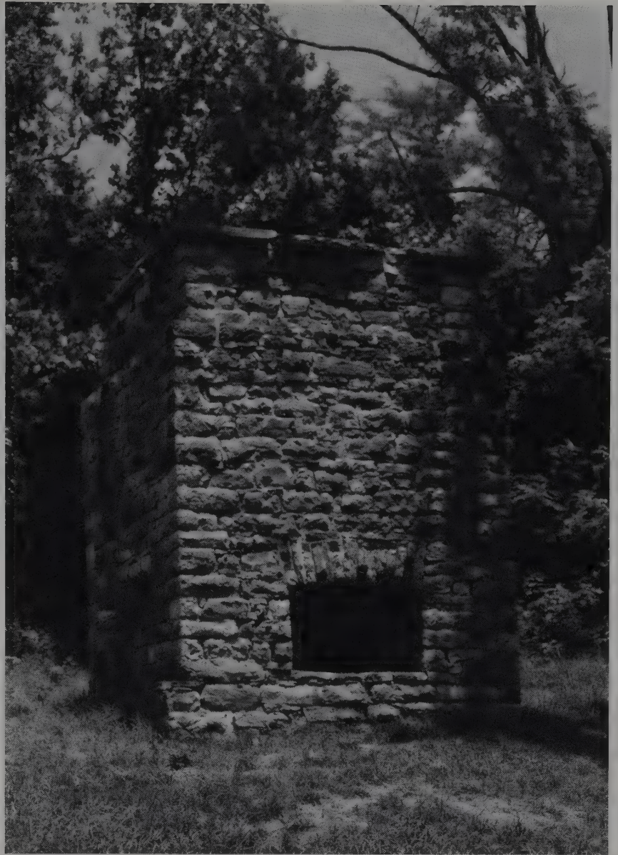
Figure 2. Morning Star silver smelter in 1988 following stabilization by the National Park Service.
