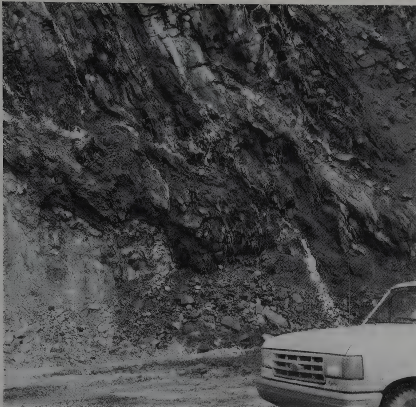
Figure 7. Schistose area in the Crystalline pit, riddled with white quartz veins, where the "Christmas pocket" (center of photo) was found.
