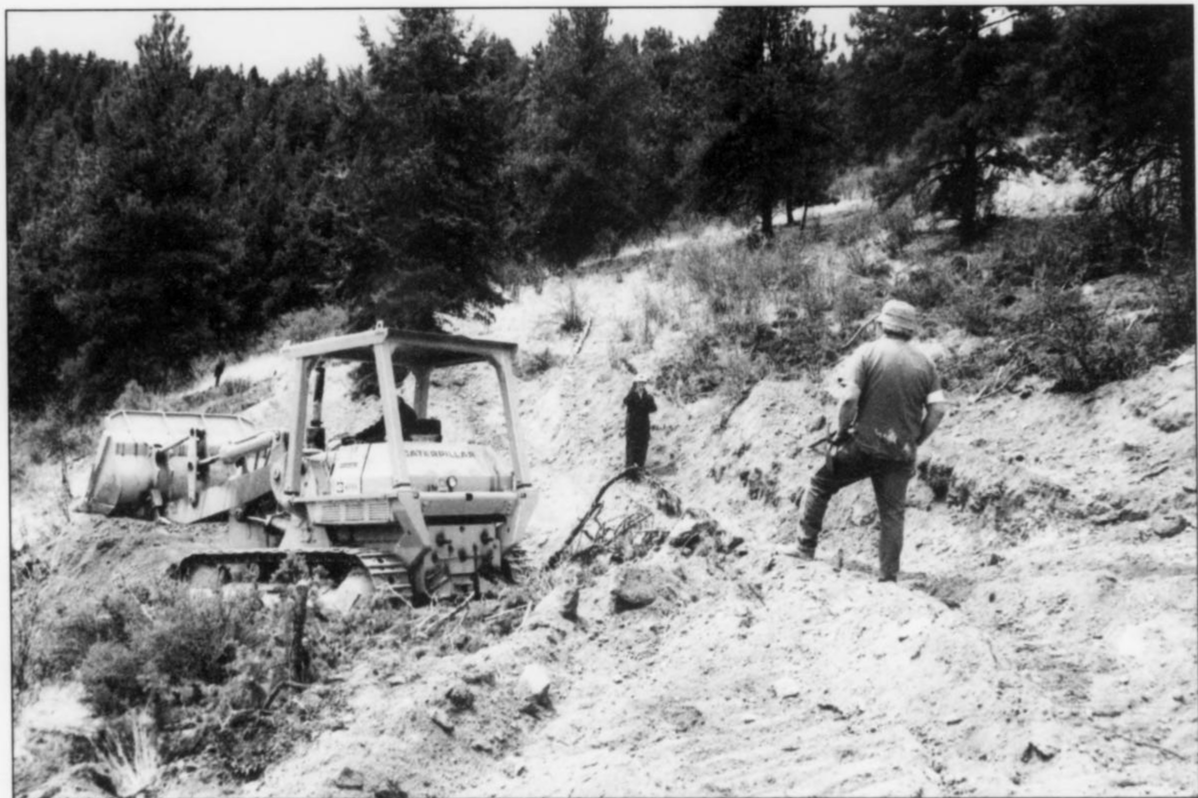
Figure 1. Bulldozing into the "Tree Root pocket" zone at the Two Point mine, Teller County, Colorado.
