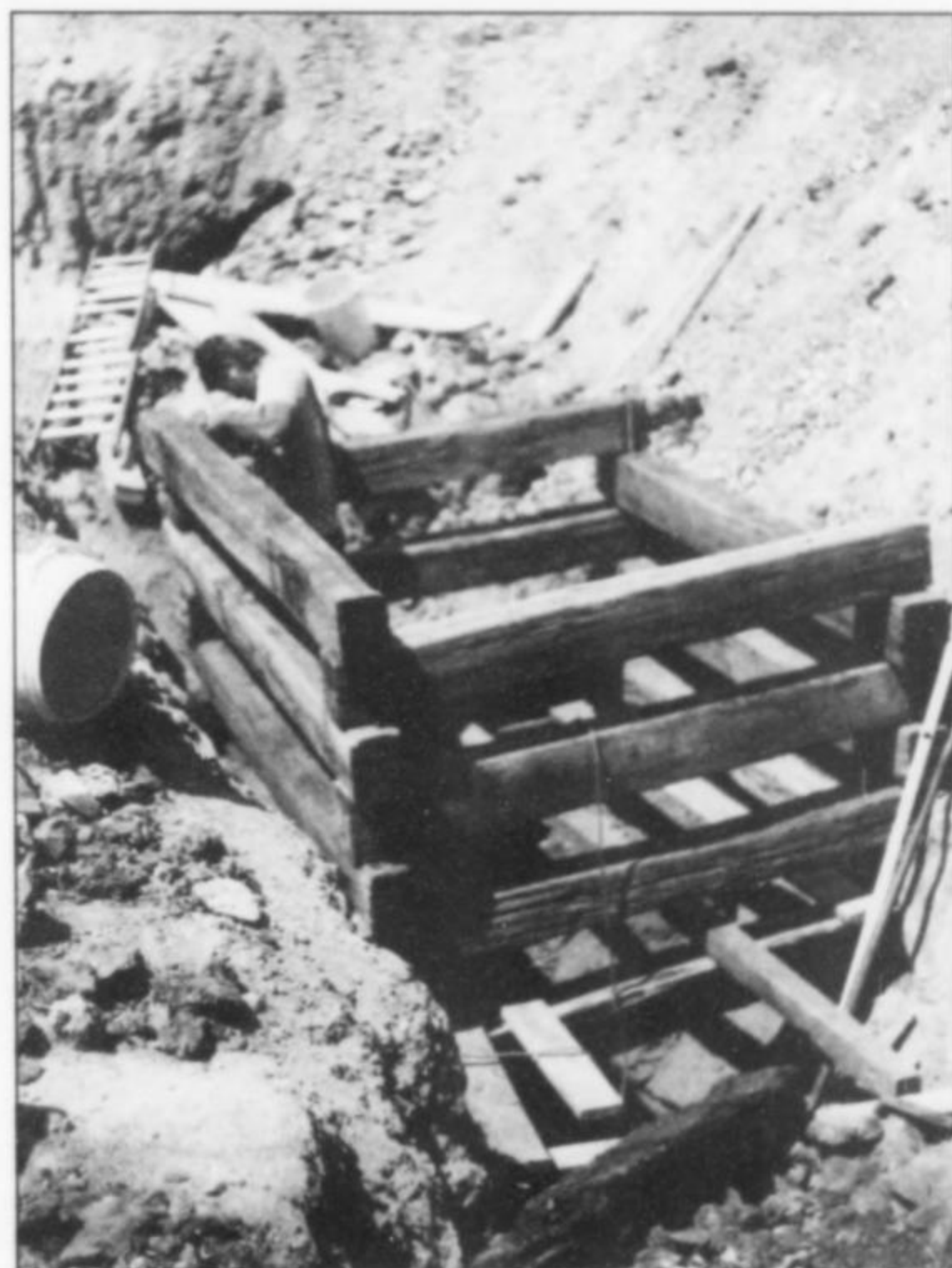
Figure 3. Rebuilding the collar at the head of the vertical shaft, Purple Passion mine.
