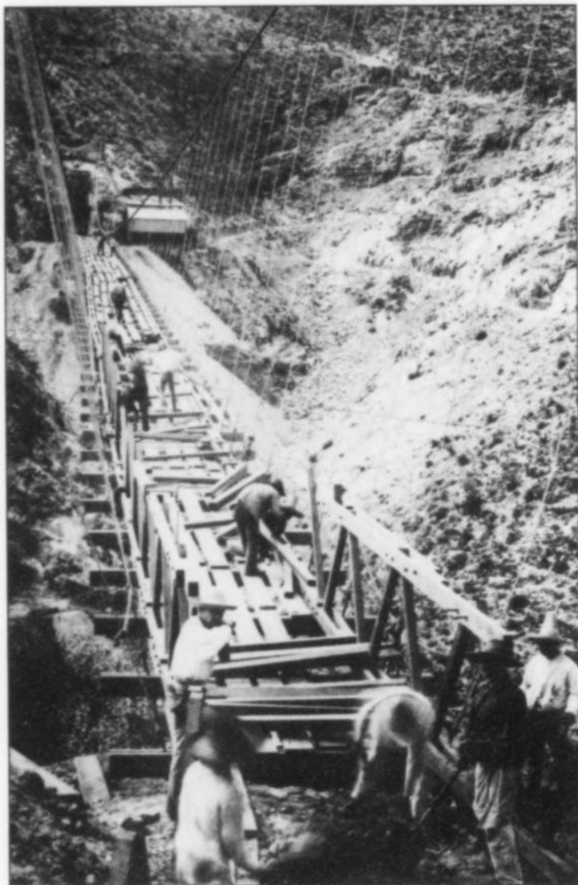
Figure 10. Constructing the deck of the Roebling suspension bridge, ca. 1892. Photo courtesy of the Mapimí mining museum and Brad van Scriver.
