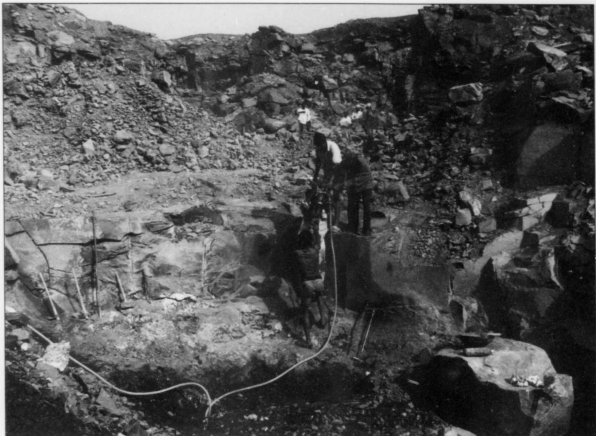
Figure 3. Drilling blast holes for the purpose of removing the overlying layer of compact aa basalt from the cavansite-producing andesitic pahoehoe horizon.
