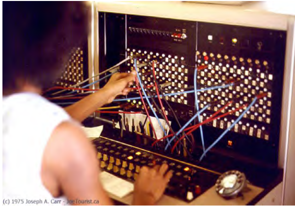
FIG. 9. A human operator physically connects a phone call using patch cables and a telephone switchboard. (photo by Joseph A. Carr, 1975)
