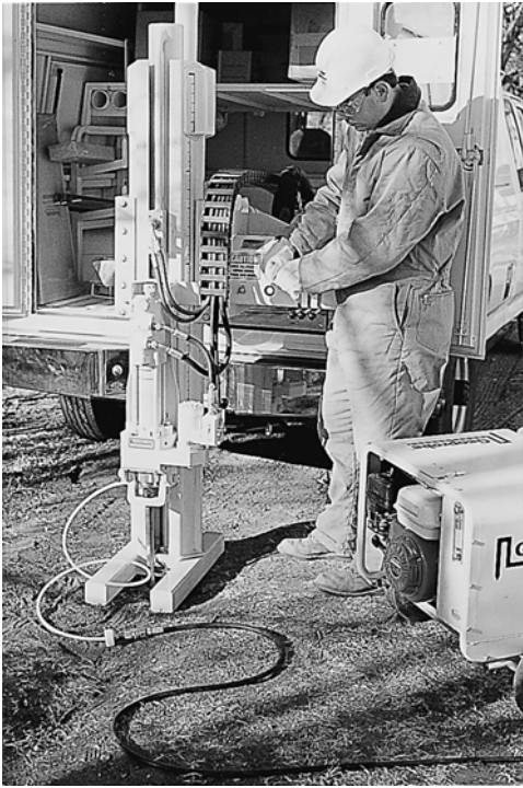
Figure 8.7 Truck-mounted GeoProbe ® for creating direct push wells for nanoiron injection. Photo is courtesy of GeoProbe ® Systems, Inc., Salina, Kansas.
