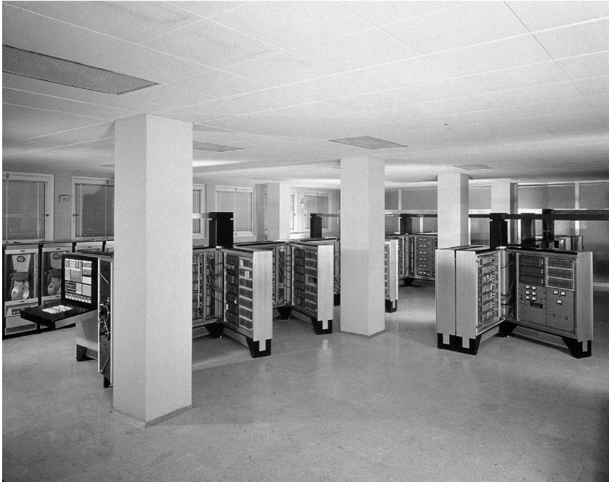
Figure 3.2 The Elea 9003 mainframe computer is a system designed by Ettore Sottsass comprised of modules of standard metal cabinets connected by a series of overhead busways. (Associazione Archivio Storico Olivetti, Ivrea, Italy).
