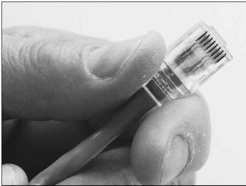
Figure 20.20 Push the RJ-45 connector into place, ensuring the cable pairs are ordered properly.
