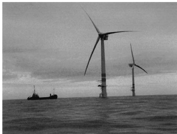
Figure 9.1.9d Located about 10 km off the coast of Arklow, Ireland, the Arklow Bank offshore wind park consists of seven GE Wind 3.6-MW wind turbines. Construction was completed in 2003. (Photo: Robert Thresher.)
