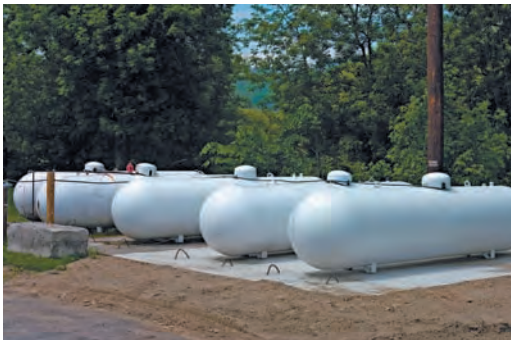
Photo 7.3 Cylindrical pressure vessels.
