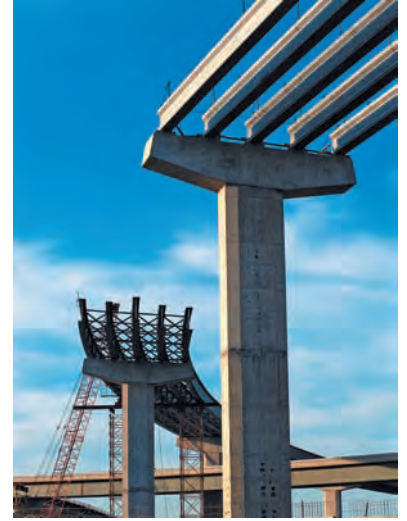
Photo 9.1 A different function M(x) is required in each portion of the cantilever arms.
