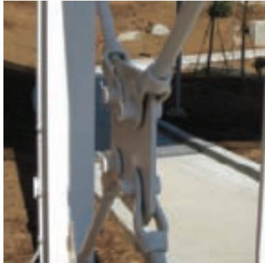
Diagonal bracing for an elevated walkway showing a clevis and a pin in double shear (© Barry Goodno)
