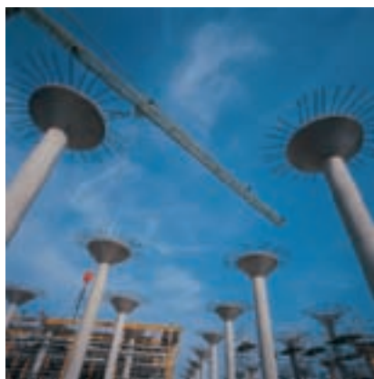
Slender concrete columns fixed at the base and free at the top during construction (Digital Vision/Getty Images)
