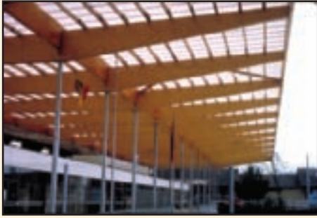
Cantilever portion of roof structure (Courtesy of the National Information Service for Earthquake Engineering EERC, University of California, Berkeley)
