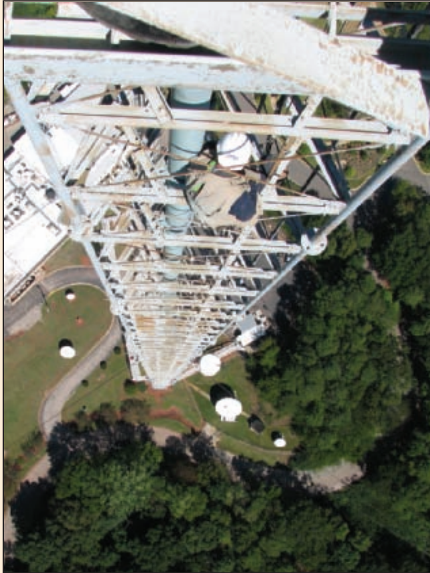
This telecommunications tower is an assemblage of many members that act primarily in tension or compression. (Photo by Bryan Tokarczyk, PE/KPFF Tower Engineers)
