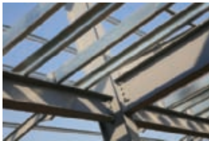
Beam-to-column connection with one beam attached to column flange and other attached to column web (Joe Gough/Shutterstock)
