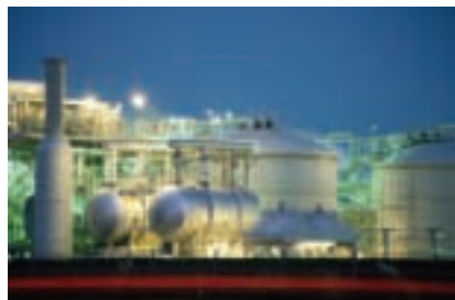
Cylindrical storage tanks in a petrochemical plant (William H. Edwards/Getty Images)
