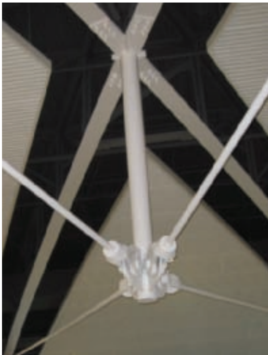
Cable and strut at typical joint of airport concourse roof © Barry Goodno
