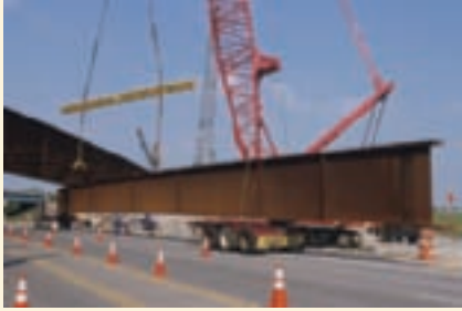
Bridge girder with overhang during transport to the construction site (Tom Brakefield/Getty Images)
