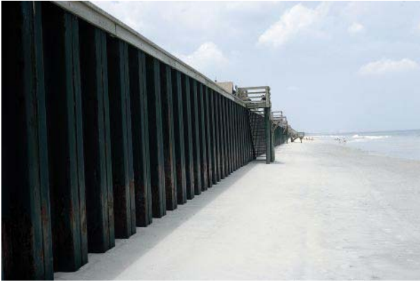
Figure 5 An example of placement loss in Virginia Beach, Virginia. The seawall was built out on the recreational beach, instantaneously narrowing the beach in front of the wall.
