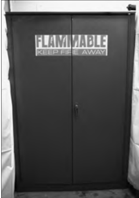
Figure 3-5: A common flammable liquids storage locker, appropriately labeled.
