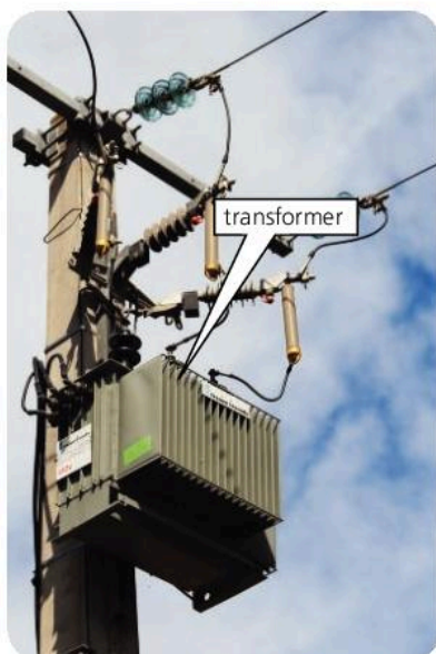
▲ A transformer connected to local power lines
