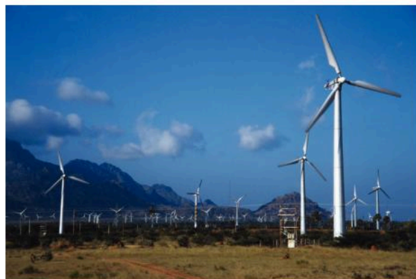
↑ Wind turbines produce electricity in India.
