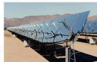
These curved mirrors use focusing the sunlight onto pipes containing water.
