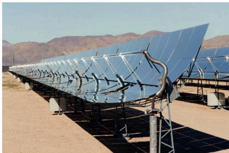
These curved mirrors are focusing the sunlight onto pipes containing water
