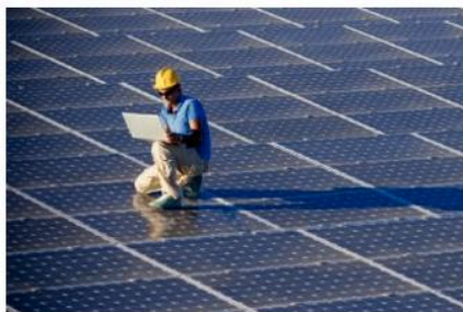
An engineer tests the output of a large array of photovoltaic cells
