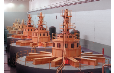
Generators at Little Goose Dam in the state of Washington. Courtesy of US Army Corps of Engineers
