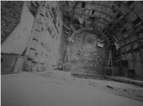
Fig. 5 Theatre auditorium: zenithal view after the fire
