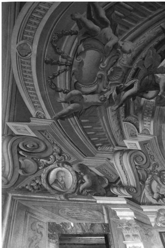
Fig. 6 A. Pozzo, Corridor of the rooms of St. Ignatius, Rome, Casa Professa del Gesù, 1682, deformation of the architraves towards the end of the corridor
