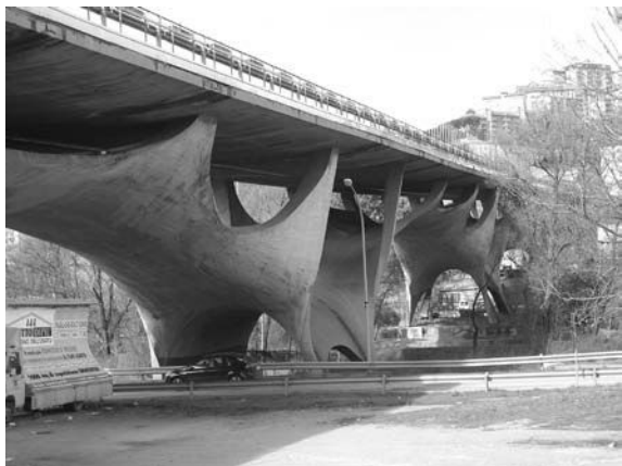
Fig. 9 Bridge on the Basenta, by Ing. S. Musmeci. Courtesy of P. Musmeci
