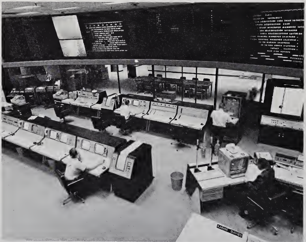
Fig. 6-17. Some of the consoles at the Space Flight Operations Facility (SFOF). Mission data are displayed for the operators on the screens and boards. (Courtesy of the Jet Propulsion Laboratory)
