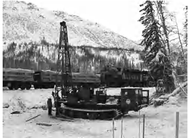
Figure 1. Rotary drilling rig used to assess shallow spillage from train derailment area at mile 262 (Photo P045; EPA).
