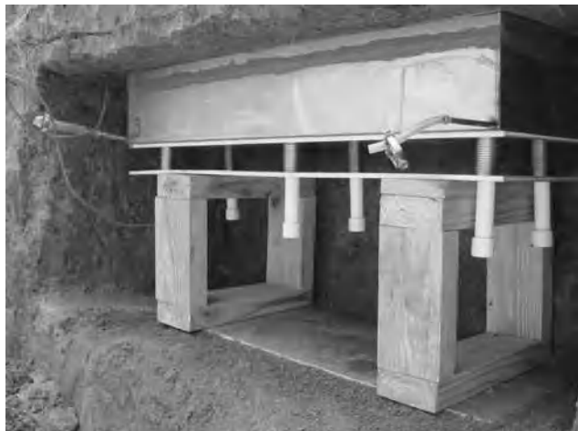
Figure 3. Rectangular cavity excavated in sidewall of the trench with nearly completed lysimeter installation.
