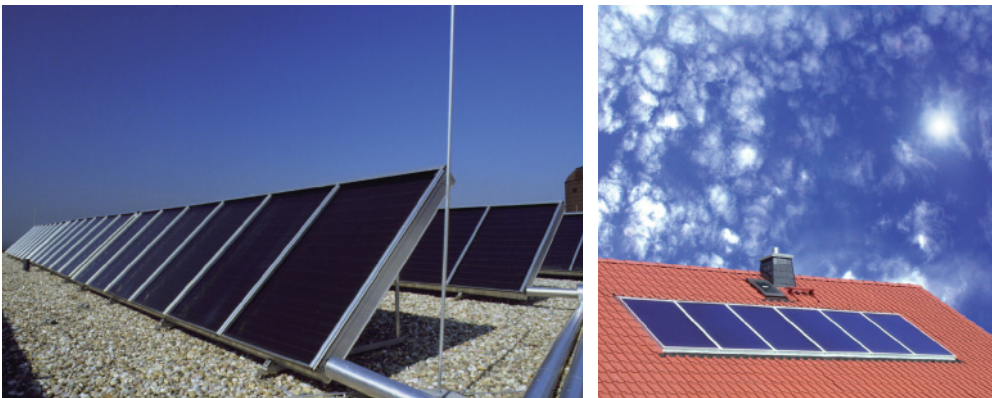
Figure 6.24 Many roofs still have space for solar collectors. Photos: www.wagner-solar.com .
