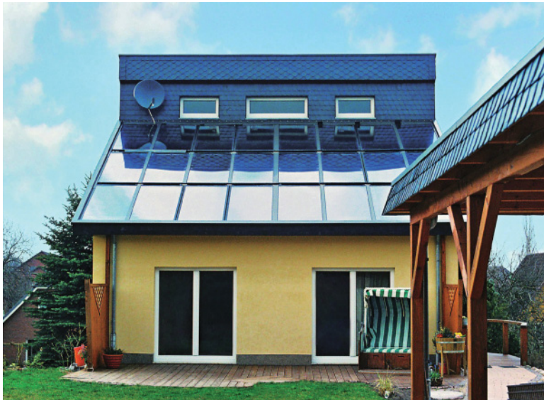
Figure 6.14 Large roof-integrated solar thermal system for heating water and providing supplementary heating. Photo: SunTechnics.
