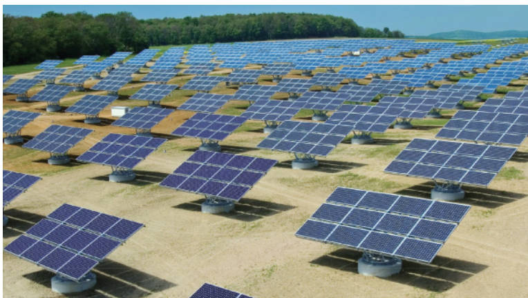
Figure 5.12 The 'Gut Erlasee' tracked solar power plant in Bavaria, Germany, has a total output of 12 megawatts. Source: SOLON AG, Photo: paul-langrock.de.
