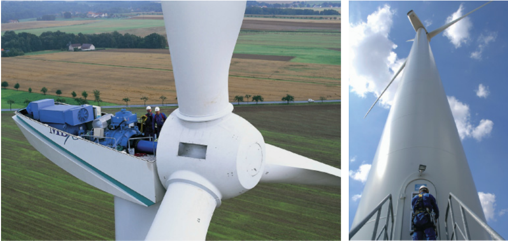
Figure 8.12 Maintenance work on wind turbines. Source: REpower Systems AG, Photos: Jan Oelker, caméléon and Stéphane Cosnard.
