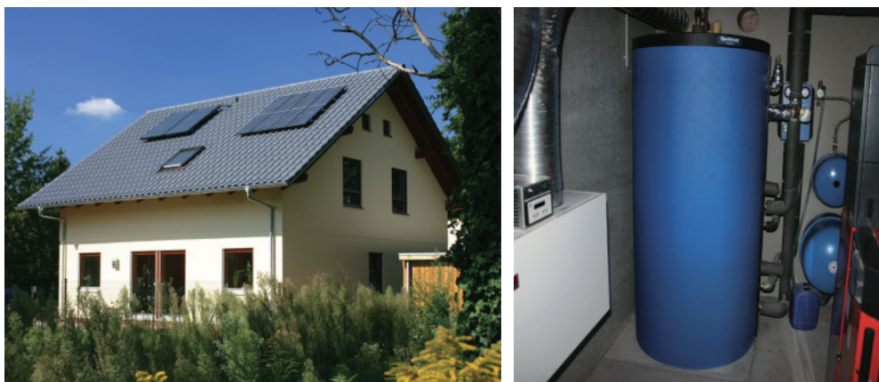
Figure 14.1 Left: Family home in Berlin with carbon-neutral energy supply. Right: Heating cellar with buffer storage tank, solar cycle pump, controlled heat recovery system and wood pellet boiler.
