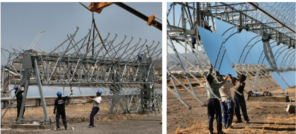
Figure 7.16 Construction of a parabolic trough collector prototype in Andalusia. Spain is currently one of the booming markets for solar power plants.
