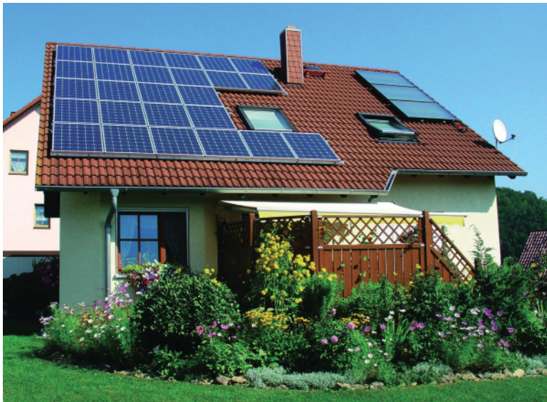
Figure 6.11 Single-family house with photovoltaic system (left) and flat-plate collectors for heating water (right). Photo: SunTechnics.
