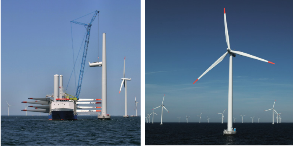
Figure 8.14 The Nysted offshore wind farm in the Baltic Sea off Denmark. Source: http://uk.nystedhavmoellegpark.dk . Construction of the wind farm. Photo: Gunnar Britse.
