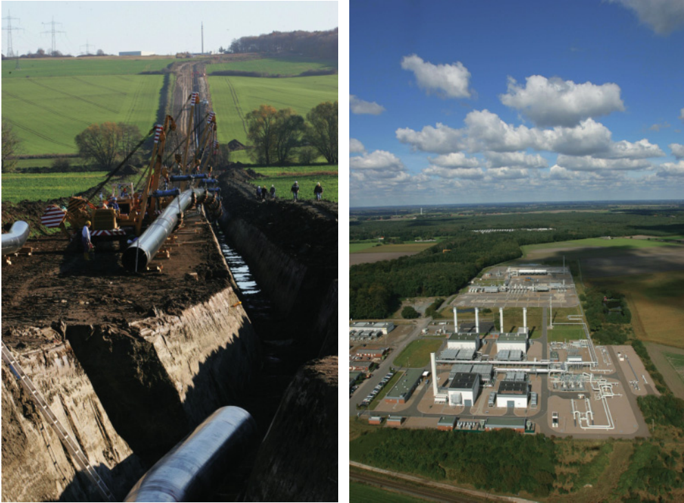
Figure 1.3 Left: Building a natural gas pipeline in Eastern Germany. Right: Storage facility for 4.2 billion m 3 of natural gas in Rehden, 60 km south of Bremen. Photos: WINGAS GmbH.
