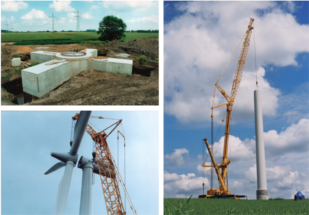
Figure 8.10 Erection of a wind turbine. Top left: Foundation. Right: Tower. Below left: Rotor and nacelle. Photos: German WindEnergy Association and ABO Wind AG.
