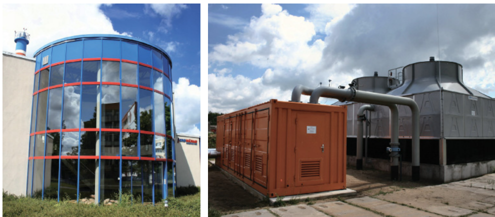
Figure 10.8 The Neustadt-Glewe geothermal heat power plant was the first plant to generate electricity from geothermal energy in Germany.
