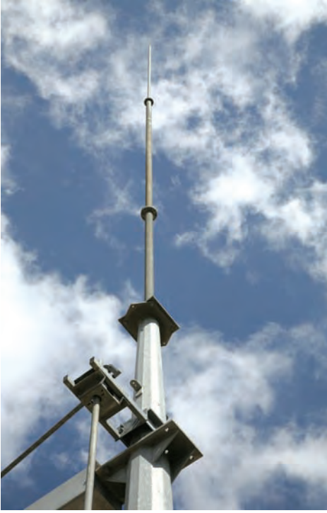
Lightning rods like this one help divert the destructive power of lightning from damaging homes and other structures.
