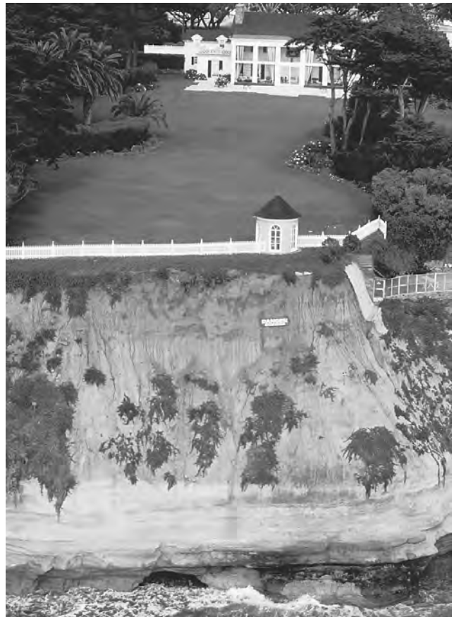
Erosive forces are pushing this cliff further back, endangering the fence and gatehouse, and eventually the main house itself. © Vince Streano/Corbis. Reproduced by permission.
