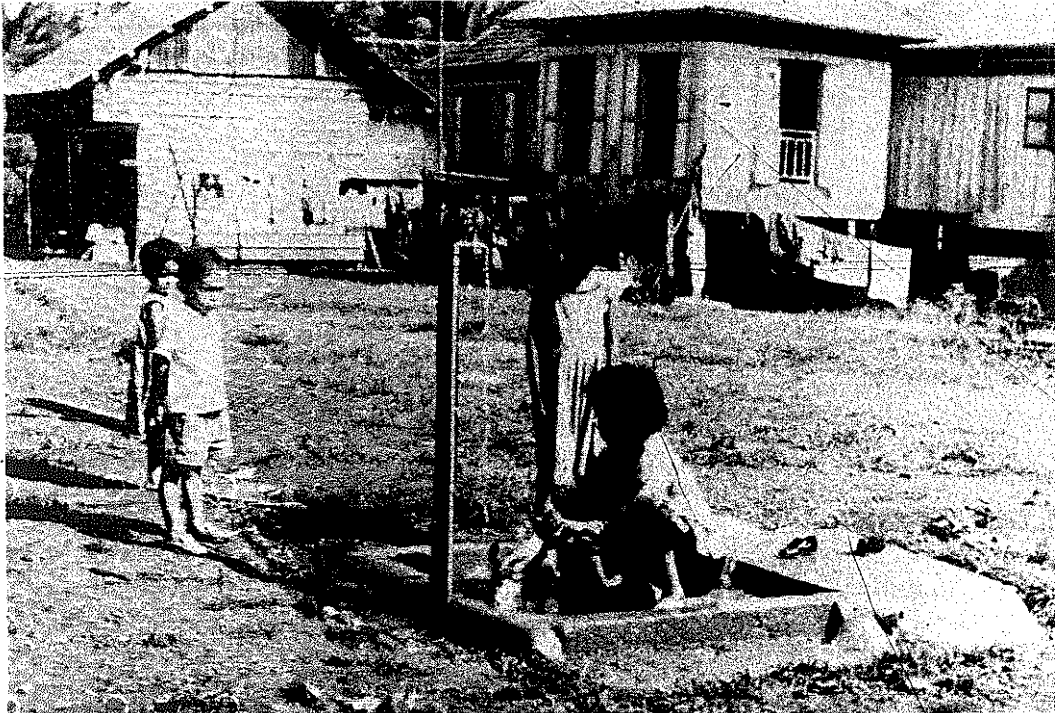
(24) Stand pipes in a W. I. member village in Sarawak, fed by gravity feed from a nearby stream, and raised high enough to allow the children to bathe under them
