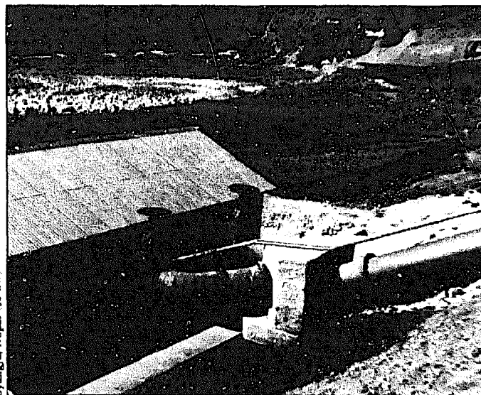
Fig. 5.20. An anchor at a bend and bifurcation at the base of the penstock.
