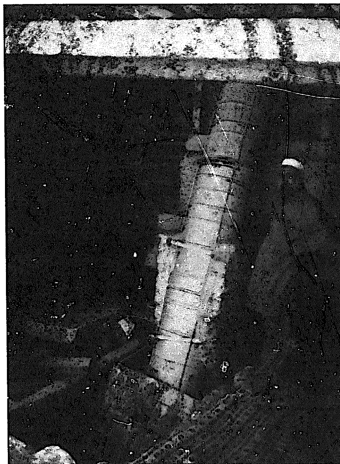
Fig. 10.57. The oil-drum penstock at the Alpuri powerhouse. The operator's bed is in the foreground.
