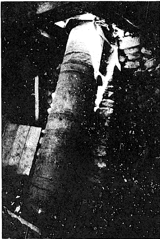
Fig. 10.53. An oil-drum penstock passes through the ceiling to the turbine, which is placed below floor level at a powerhouse at Llllonai (Fig. 10.56).
