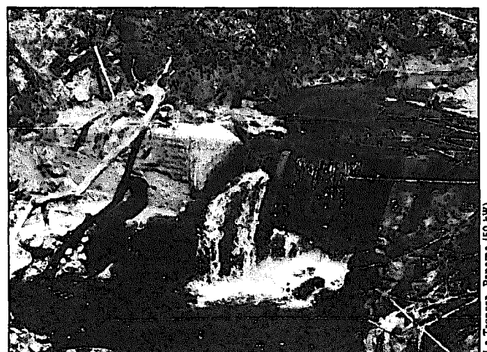
Fig. 5.39. Even before an opening for the penstock pipe could be made through the concrete intake structure to the left of the weir, flows had already seriously undermined the structure and completely backfilled the intake and area behind the weir. The design did not include an opening behind the weir for sluicing out the accumulated sediment behind it.
