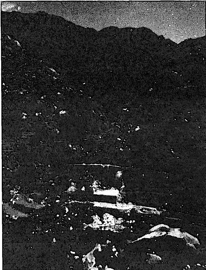
Fig. 10.40. The Barkalay powerhouse uses excess water available from an irrigation canal that cuts across the slopes a short distance uphill. Two other hydropower schemes are located farther up this same valley (see Figs. 10.51 and 10.58).
