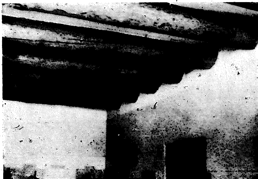
Figure 86. The large and small ends of the ceiling timbers (vigas) are alternated to provide a balanced appearance.
