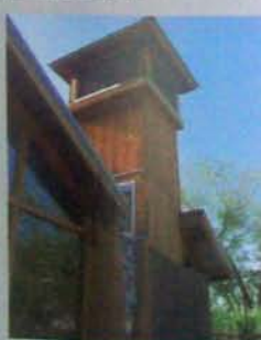
Roof water from the addition is channeled down a tiled downspout next to the cooling tower and into a pumice-filled planting bed.
