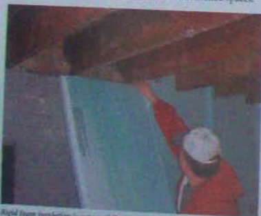
Rigid foam insulation is cut carefully around floor joists to seal the rim joint and basement walls.
