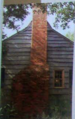
The house's natural ventilation was increased without altering its historic appearance by inserting small screened gaps between horizontal siding boards.
