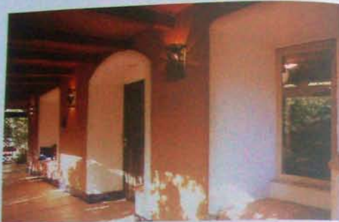
If you are changing exterior wall finishes, it's relatively easy to replace the whole window, rather than just the sash.
