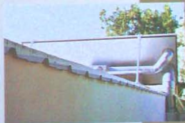
Warm air is ducted from the solar panels into the house.
