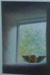
Incident light reflected off the light-colored, splined joints of a straw-bale wall makes the opening seem larger.
