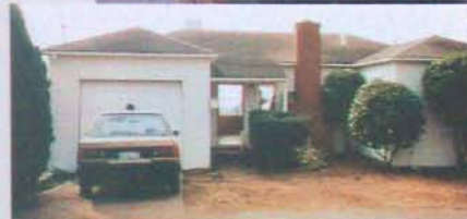
A neglected rental home for many years, Kelly saw the home's potential.
