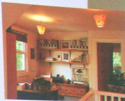
Sometimes subtraction is a plus; here, removing some walls adds natural light and ventilation.
