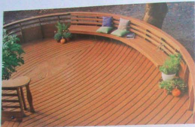
Like any relatively new product, installation of plastic composite decking differs from that of wood decking.
