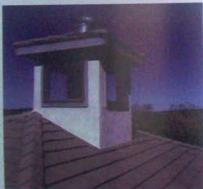
A cupola allows warm air to escape. A wind-driven turbine aids an extra boost.
