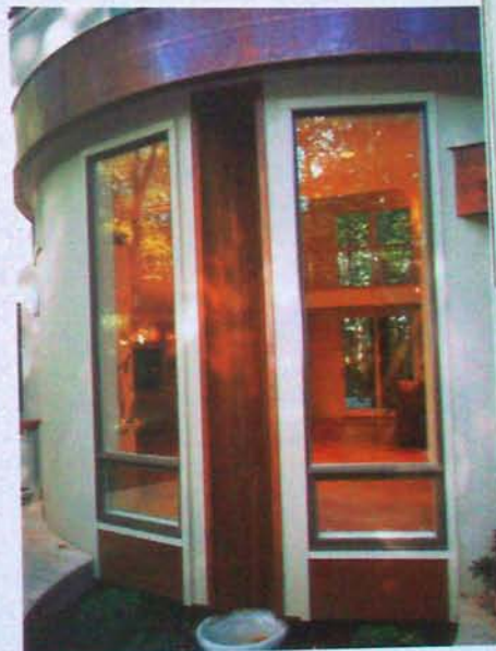
This unique downspout guides roof water to a splash bowl, which protects against soil erosion and overflow, watering nearby plants.
