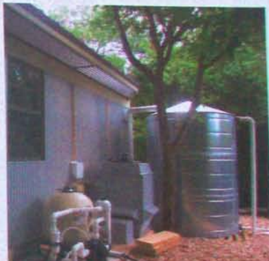
This cistern stores rainwater runoff from the roof until it is needed for landscape irrigation during dry Austin, Texas summers.
