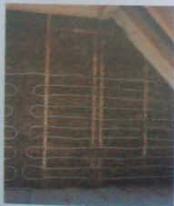
Hydronic heating in the walls is common in Europe, but a relatively new practice in the United States.
