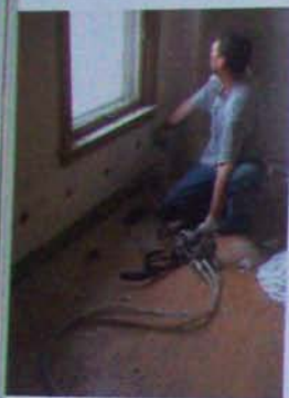
Installing spray-foam insulation in wall cavities through holes in the interior plaster.
