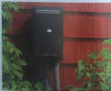
Tankless water heaters are small. In climates where temperatures don't go below 37°, they can be mounted outside.
