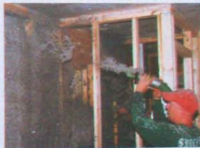
Cellulose insulation, bound with water-based glue, can be blown into wall cavities. Excess insulation is scraped off, leaving a flat layer that fits snugly around the studs, electrical cables, and box.
