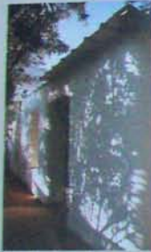
A metal roof covers the tops of some new straw bale walls.
