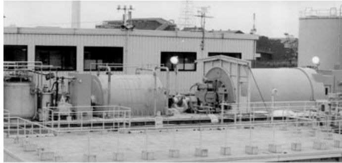
Fig. 8. Superconducting generator on the stage of the Super-GM testing center (from left to right: liquid-helium dewar, superconducting generator, driving motor). (By courtesy of Super GM.)
