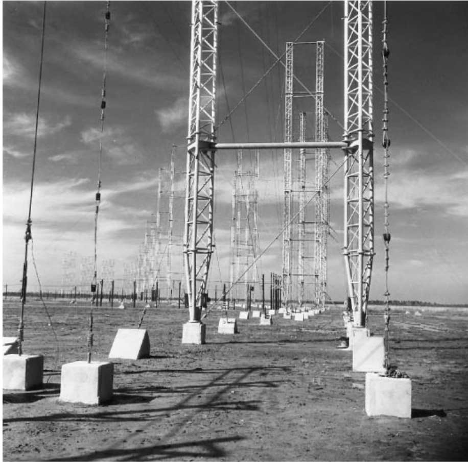
Fig. 1. High-frequency broadcast antenna arrays at the Voice of America's Edward R. Murrow transmitting station near Greenville, NC. Guyed masts up to 100 m support arrays of folded dipoles in front of wire reflecting screens. Courtesy USIA International Broadcast Bureau.
