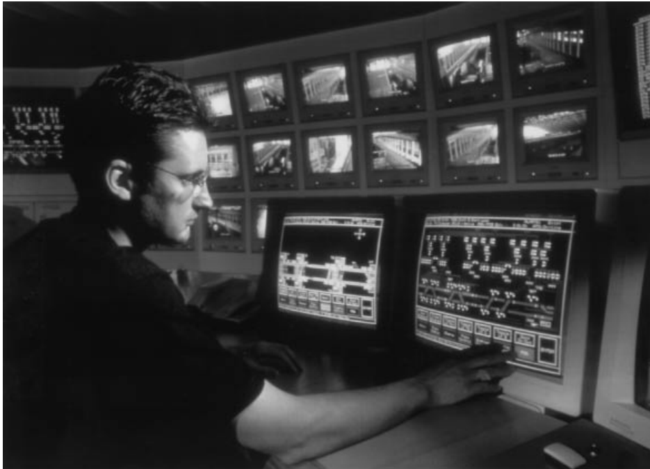
Figure 2. Automated guided transit system control center at Frankfurt/Main Airport, Frankfurt, Germany. Photo credit: ADtranz.
