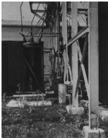
Figure 2. 14.4 kV, 600 A, oil circuit breaker (courtesy of Marcel Dekker).
