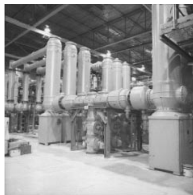
Figure 4. A typical 230 kV gas-insulated substation. (Photograph courtesy of Ontario Hydro.)
