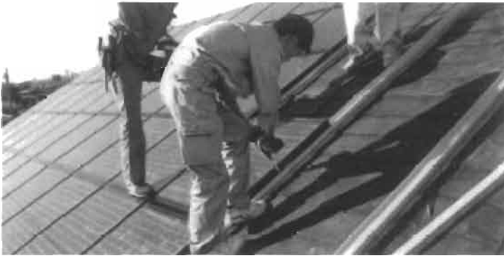
Figure 10 Installing a sloped PV roof. Source: IEA Task VII PV Database. © MSK Corporation. Reprinted with permission.
