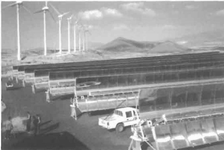
Figure 17 Example of a concentrator array field. Seven of the fourteen parabolic troughs constituting the EUCLIDES demonstration plant installed in Tenerife are shown in this picture ( 480 kW_p ). The plant includes a monitoring station and seven inverters, one for each pair of arrays. The project is supported by the JOULE-THERMIE Programme.
