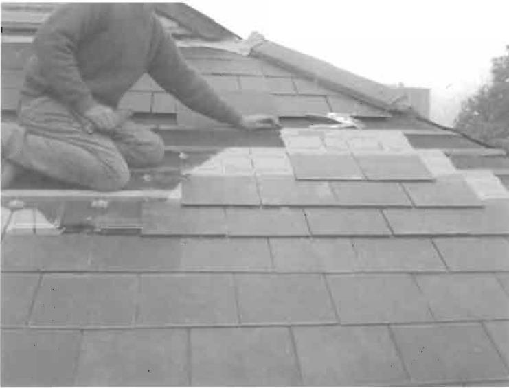
Figure 10 The uniform appearance of the thin film solar cells means that the four rows of Electra-slates being installed in Cardiff are almost indistinguishable from the rows of standard synthetic slate above and below them. The glass section at the top incorporates the interconnections and is covered by the row above when installation is complete.
