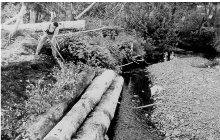
Figure B. A physically stabilized streambank, with a worker replanting native alder trees, which fix nitrogen and help to further stabilize the streambank with vegetation. (Photo by P. Swartzbart.)
