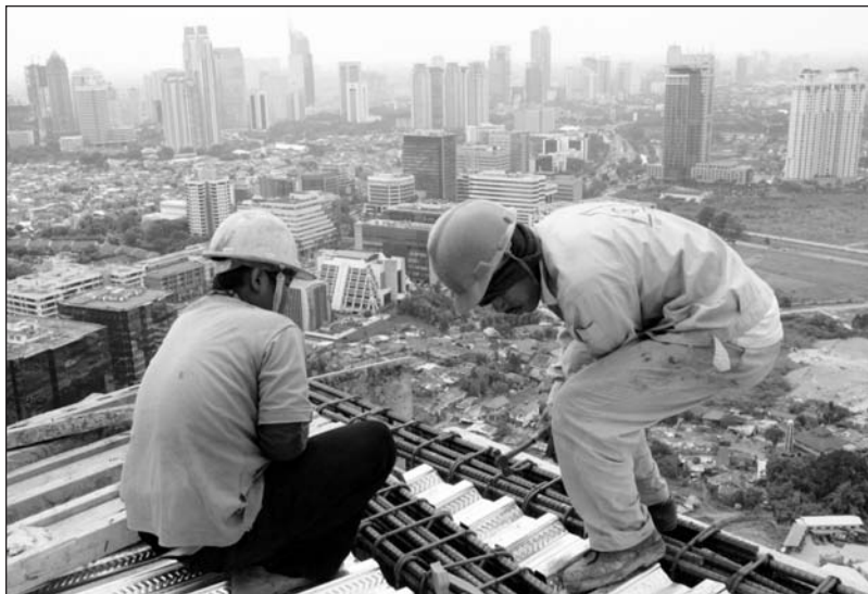
Construction workers build a new apartment building in Jakarta, Indonesia, one of Asia's fastest-growing megacities. (Supri/Reuters/Landov)
