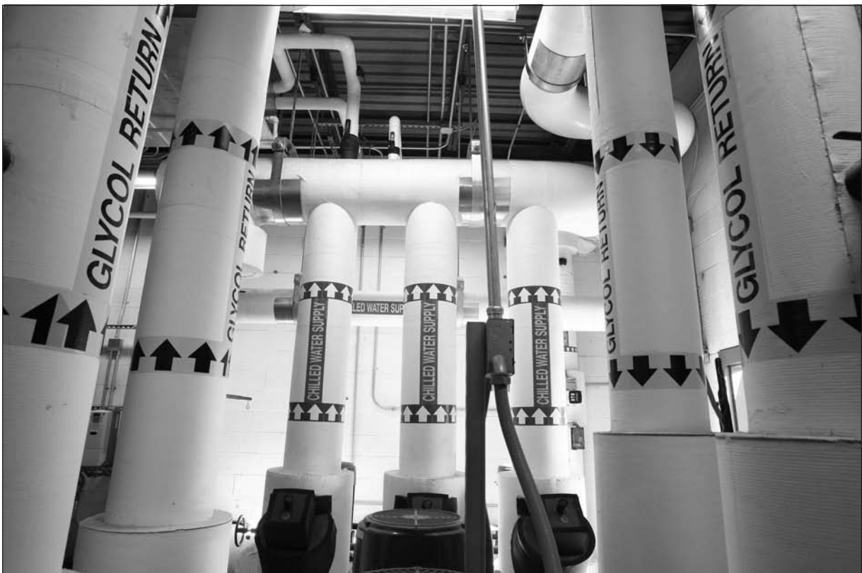
On Dyess Air Force Base, in Abilene, Texas, a chilled glycol slurry is used to cool buildings in an effort to decrease the base's environmental footprint. (Ralph Lauer/MCT/Landov)
