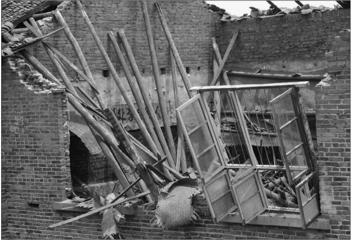
This middle-school classroom in Lianyuan, China, collapsed as a result of termite damage in May, 2007. Increased global warming may increase the population and range of these pests. (Reuters/Landov)
