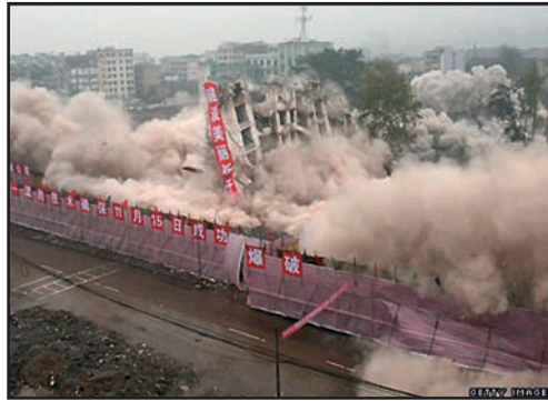
Figure 5.1 A block of buildings is demolished in Chongqing, China, to clear land that will be submerged by the Three Gorges Dam. (Getty Images, 2007)
