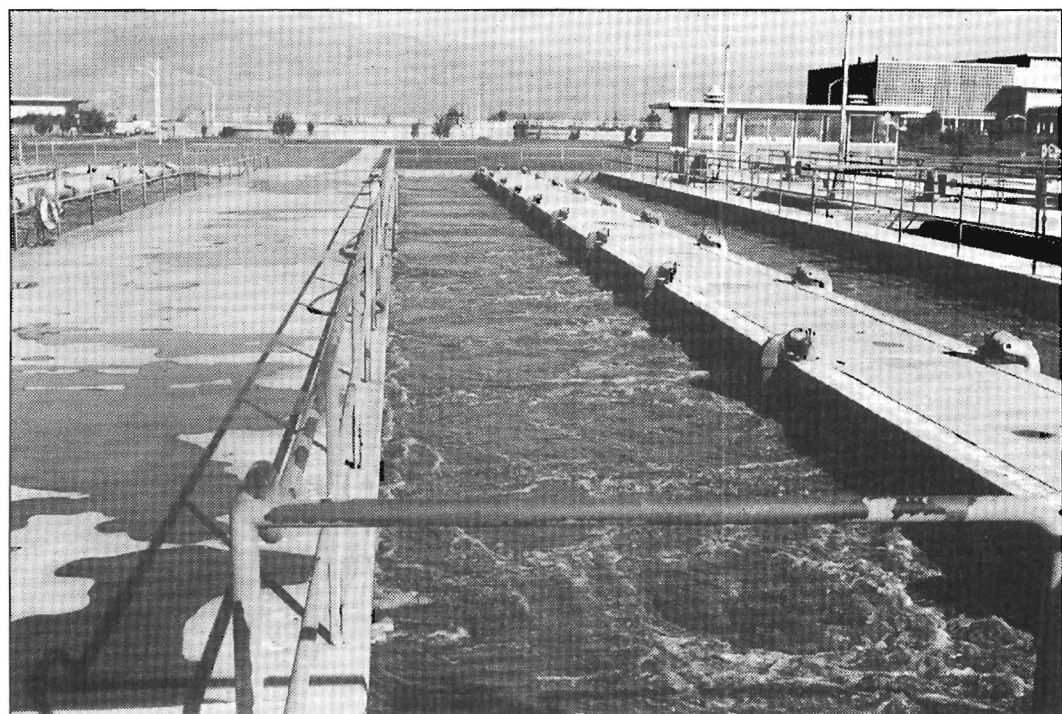
Photo 6.1 A typical "plug flow," diffused-aeration tank for conventional activated sludge.
