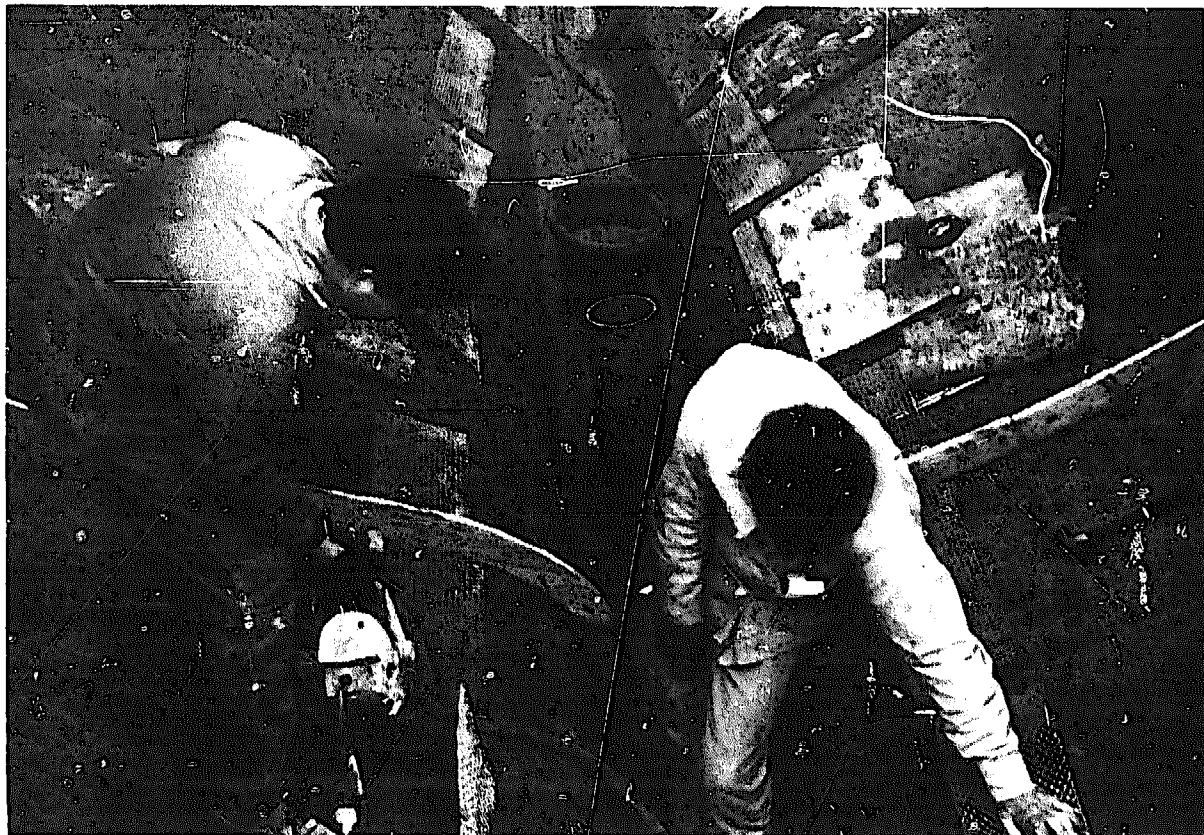
Figure 4-18. Steel and ballast keel being poured. Note scrap steel embedded in mortar mix, and vibrator being used. Wooden shapes are shutters for bulkhead grounds which can be seen meshed up in upper part of the photograph. Folded panels of mesh each side of keel are lapped across centre line after ballast is poured, tied together and finally plastered over
