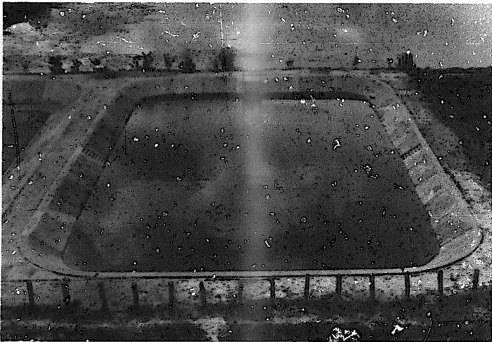
Protected sloping wall filters, Kranuan, Thailand (background pre-sedimentation pond).
